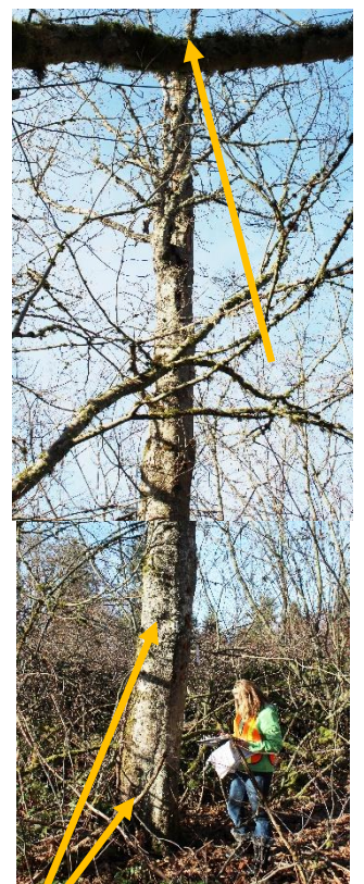
7489 Cottonwood, Previous top failure, column of decay, cavities of decay, dead branch's,
